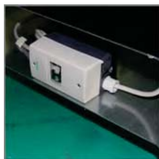
Boitier de commande Electric panel board
